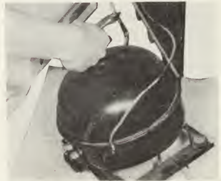
17-25. Pinching the suction line prior to wrapping it in cloth and breaking it. (Philco Corp.)
